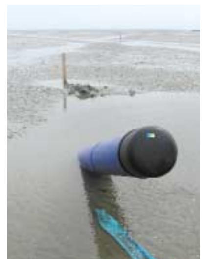
The pipe end in the mud-flats, which were installed with the "plow"
