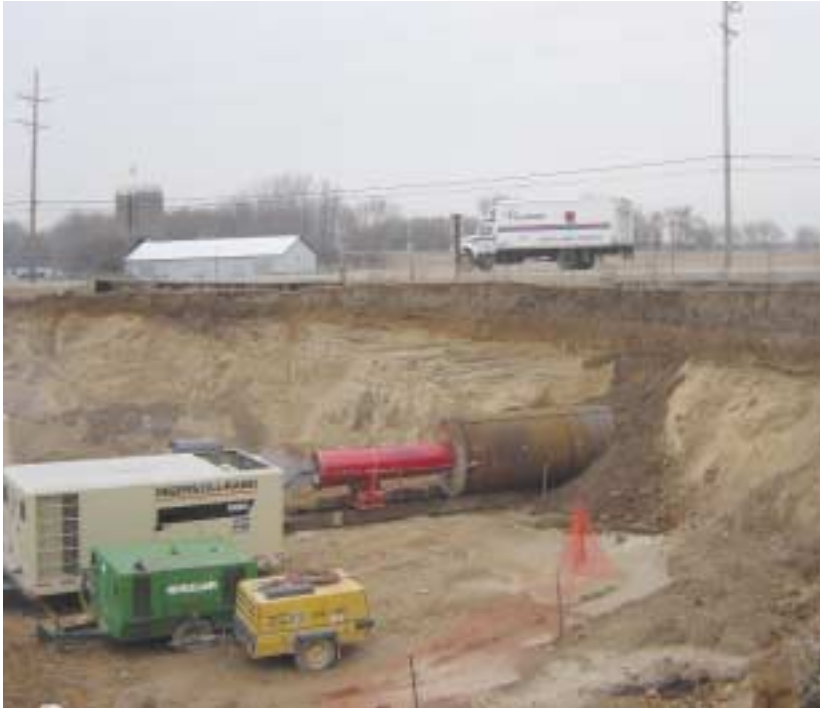
Once in place, the casing ND 2000 would facilitate the expansion of a gravel operation. A conveyor system will be placed through casing to carry gravel from a new pit on one side of the highway to the crushing facility on the other.
