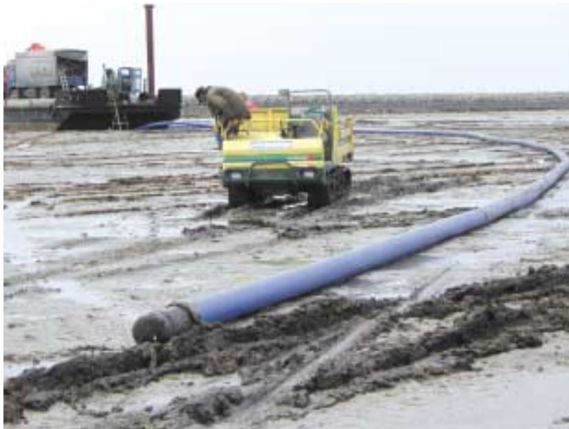
The pipes are ready for installation. The pontoon in the background with the bore rig.
