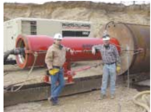
Powers Lake Construction prides itself on quality work and attention to detail. Here Powers Lake Construction President Mark Karow (left) and Project Manager Noel Karow pose next to the world's largest pipe rammer.
