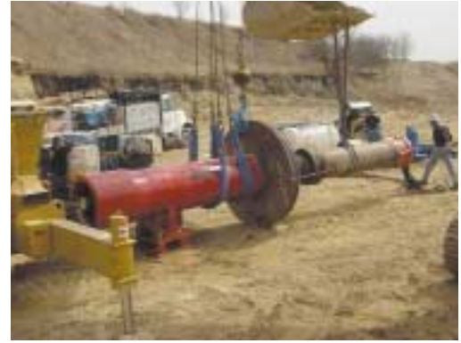
Two pipe rammers were used on the project. The Grundoram Taurus started the project then moved to another jobsite. The Grundoram Apollo was brought in to finish the job.
