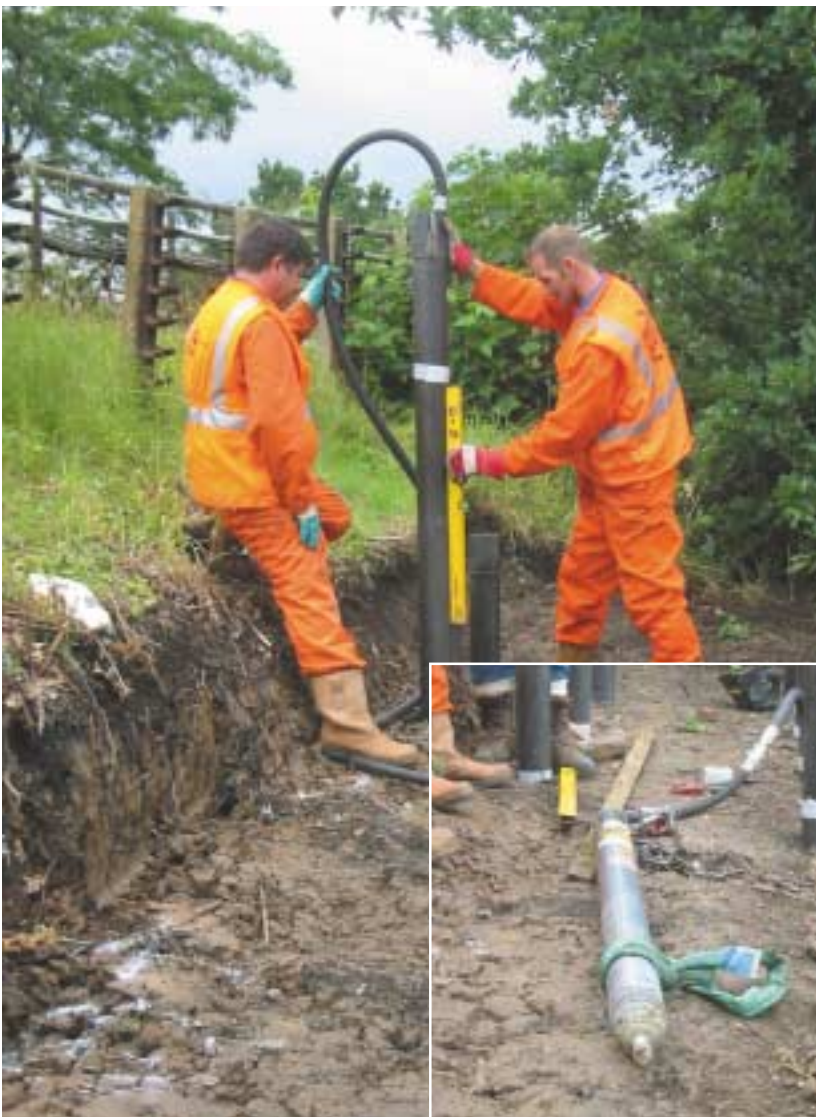
The Operators ensuring the pile is driven plumb by using a spirit level
