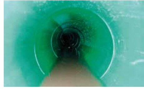
The hydraulic capacity is maintained.
