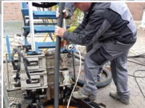
Insertion of heat exchangers.
