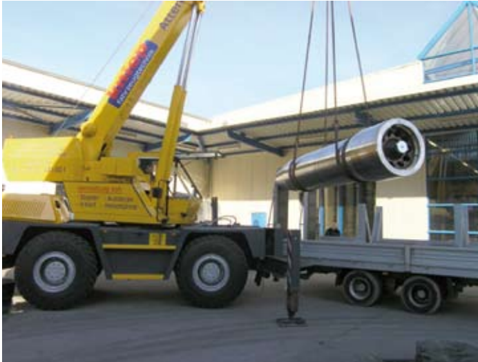
A 20-t crane had to be hired for the transport of the huge ramming machine from the factory to the test stand.
