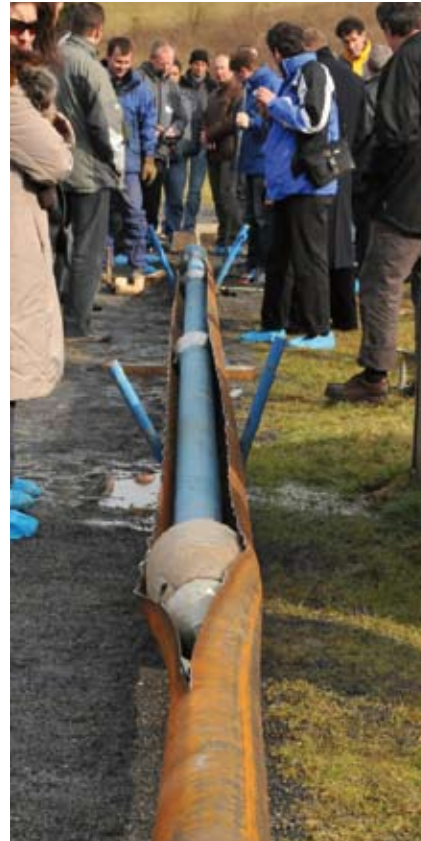
Demonstration of the GRUNDOBURST 400G above ground: Cutting of a steel pipe (old pipe) and simultaneous pulling in of the new ductile iron pipe.
