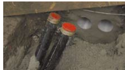
The installed long distance heating pipes with both core bore holes in the cellar.
