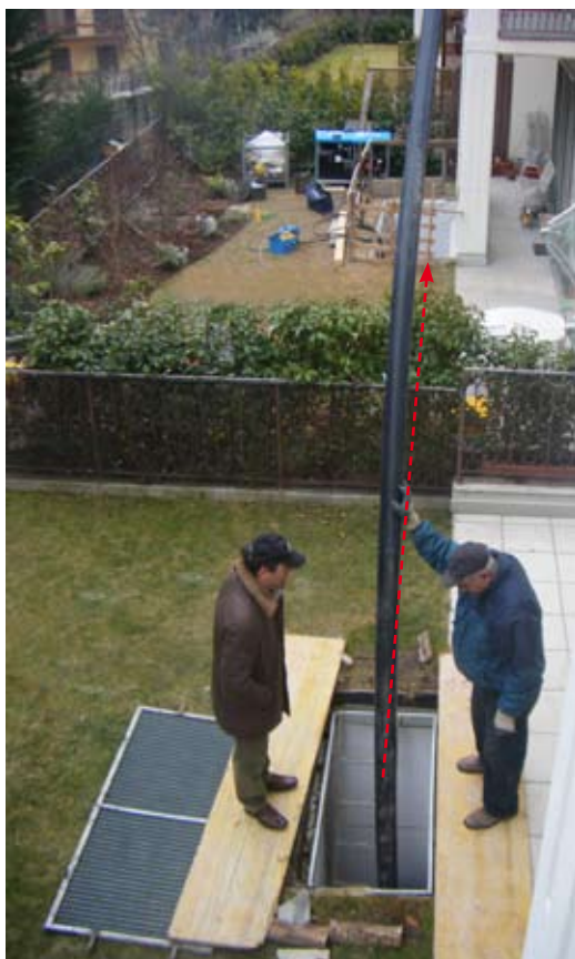
The GRUNDOPIT during the installation of the HDPE pipe ND 110 from the reel.
