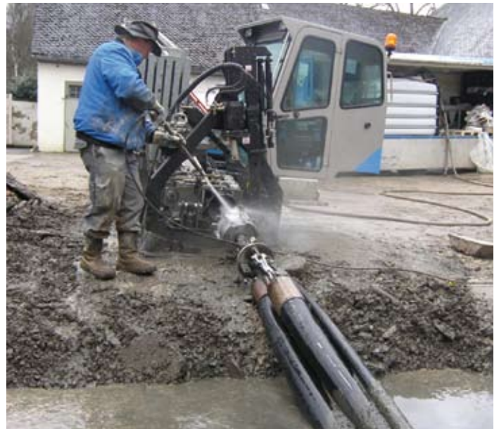
The Grundodrill 15 XP required only half an hour for the remaining 20 metres.
