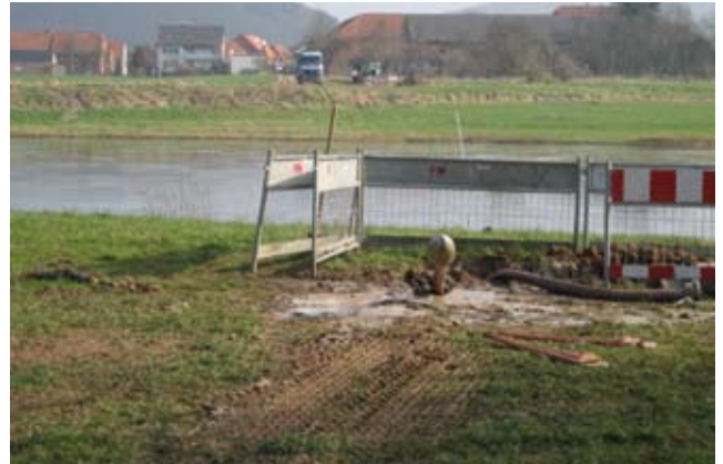
River Weser with bore rig in the background and the push head at the front.
