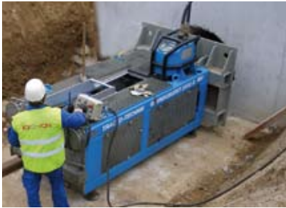
The machine pit is used in both directions. After completion of the first bursting section the GRUNDOBURST is used for the second bursting section in the opposite direction.
