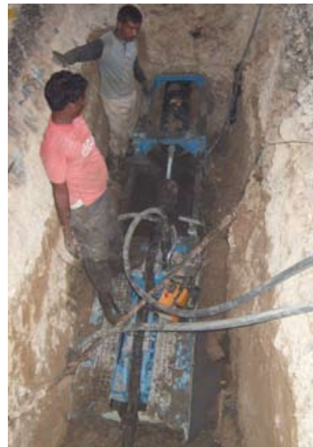
Target reached: The 355 mm PE-pipe is pulled through the telescopic frame of the GRUNDOBURST.
